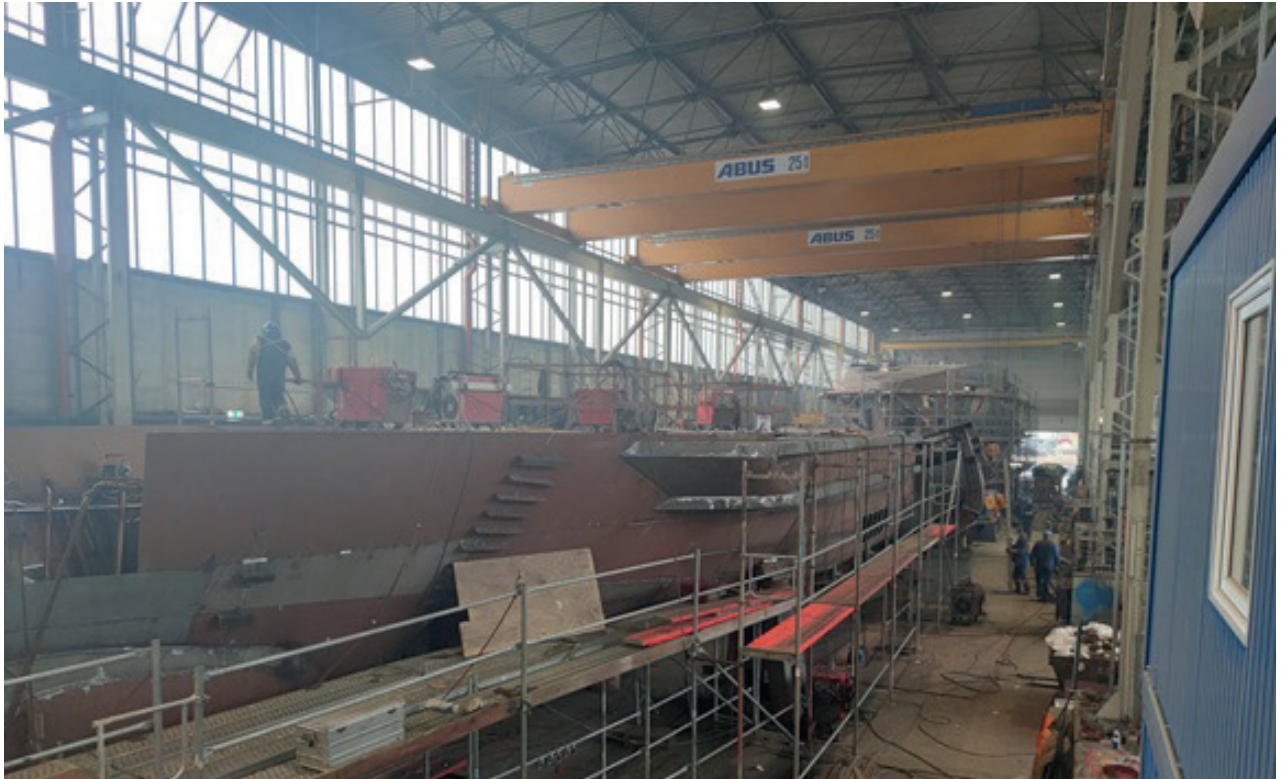
The hull of the »Grasbrook« during construction in the shipyard hall in Tangermünde
